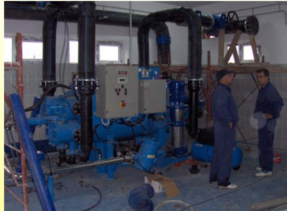
Photo 5 –MTG device for water treatment
