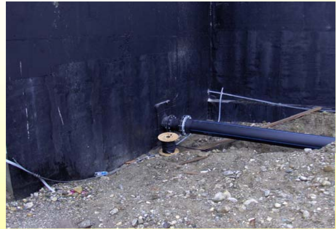
Photo 2- Input of supply pipeline into a reservoir
