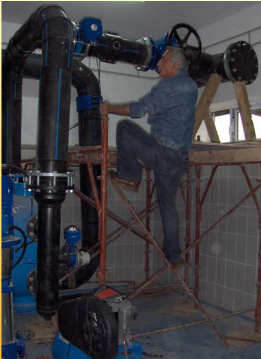
Photo 6 – part of the equipment in the filter station
