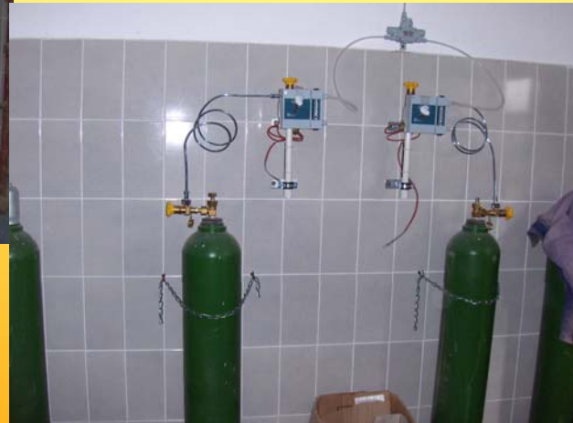
Photo 8 – Equipment for chlorine
