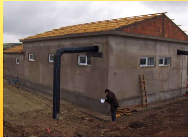
photo 4-Filter object with chlorine station
