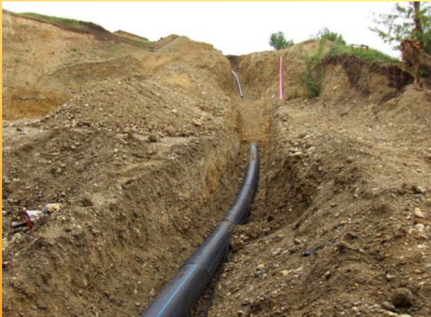
Photo 3-Supply pipeline from a filter station to a reservoir
