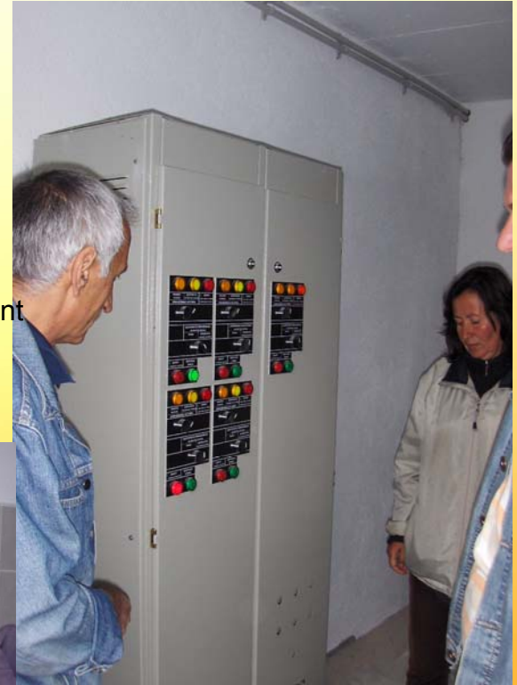
Photo 7 – commanding premise with filter station
